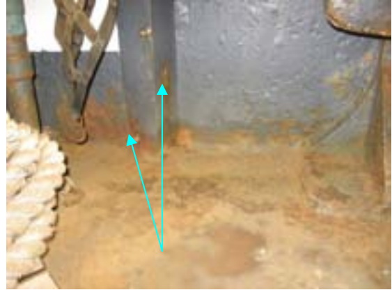
Superstructure with holes
