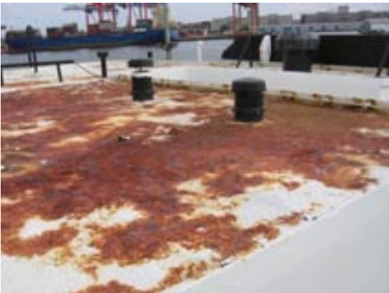
Housetop coating failure and active corrosion
