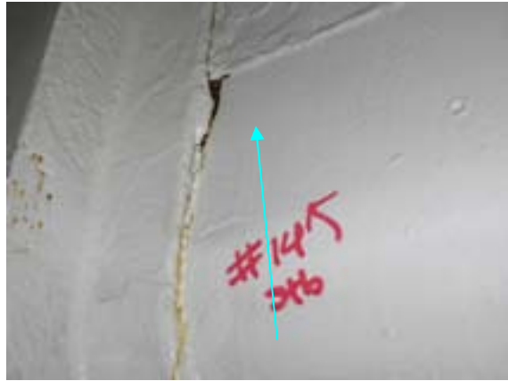
Cracked weld at frame
