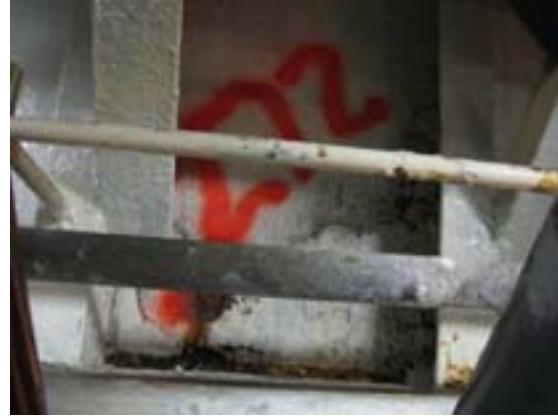
Corroded shell plating
