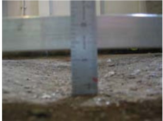
Buckled down – 1-3/8" depth
