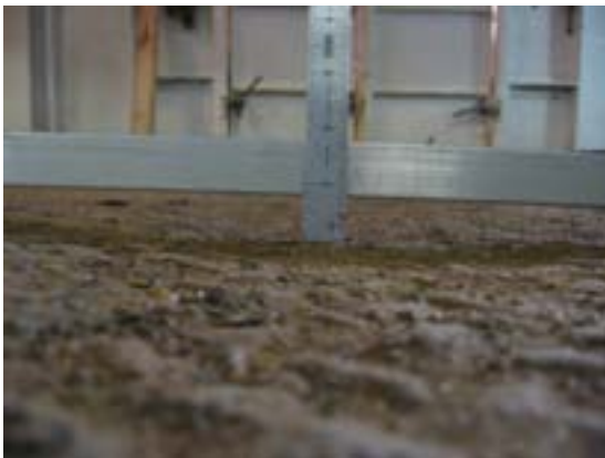
Buckled down – 13/16" depth
