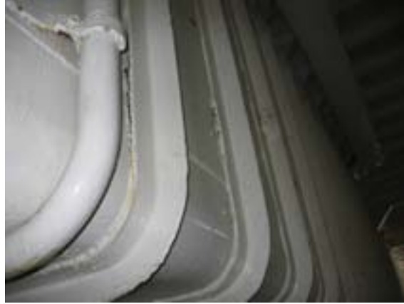
More cracked welds
