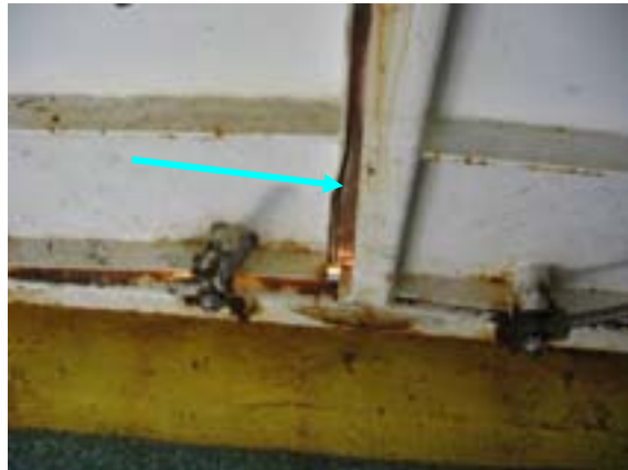
Bent watertight passenger loading door
