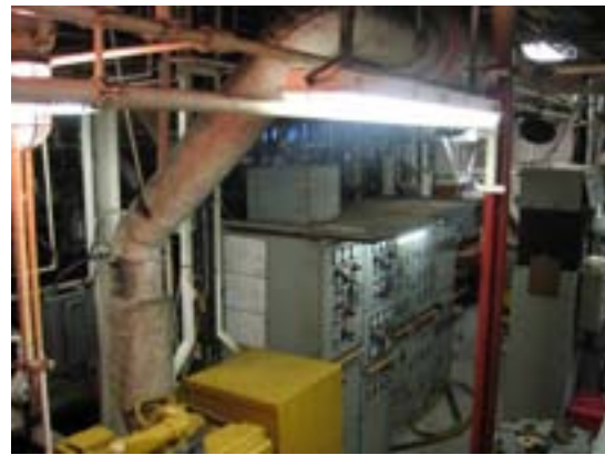
Main electrical distribution panels
