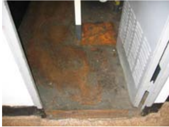
Wasted steel in salon deck
