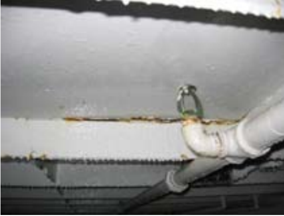
Cracked weld at deck
