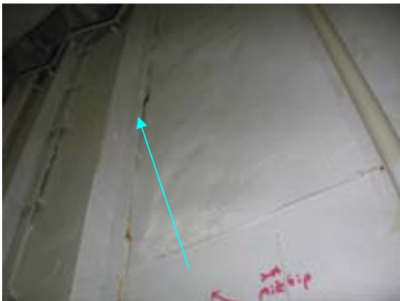
Cracked weld – buckled bulkhead
