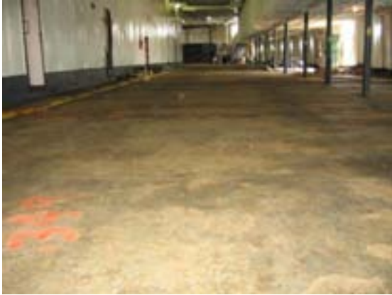
Wasted steel and coating failure
