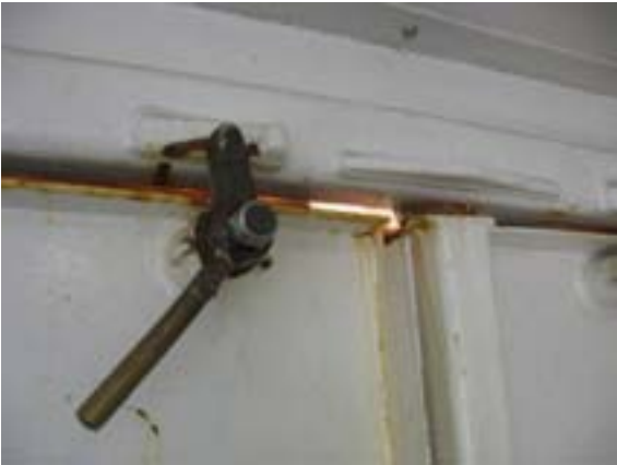
Watertight loading door will not close
