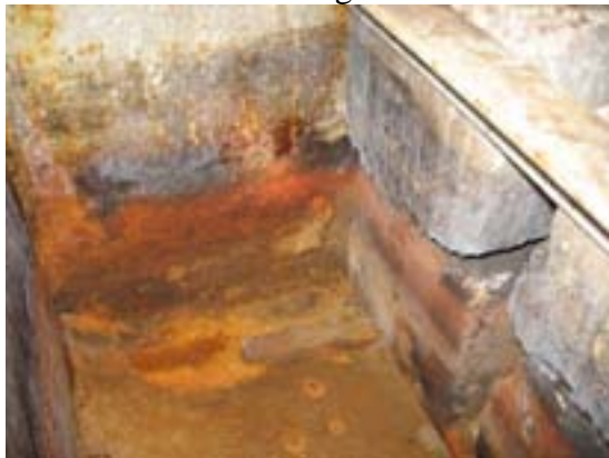
Wasted bottom plate next to lead ballast
