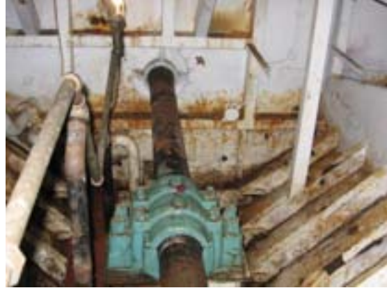
Coating failure and wasted frames
