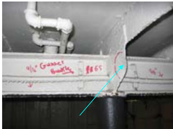
Example of buckled gusset
