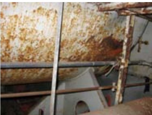
Corroded black water tank
