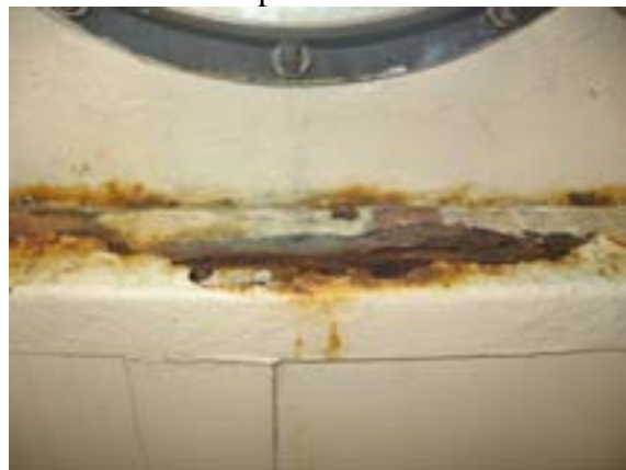
Corroded steel under porthole
