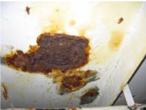
Deck wasted through in head at sink
