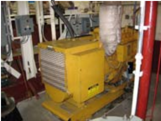
New AC Generator
