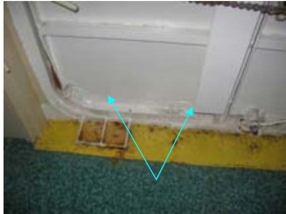
Watertight door missing dogs
