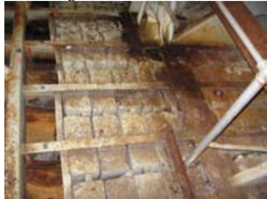
Lead ballast blocks
