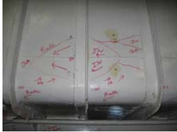
Buckled bulkhead - starboard aft
