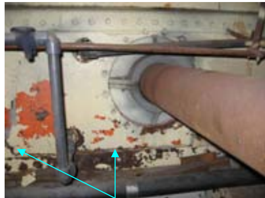
Failed Bulkhead gasket
