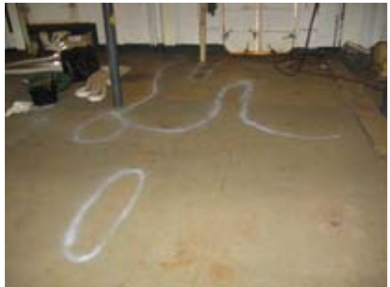
Outline – main deck buckled up
