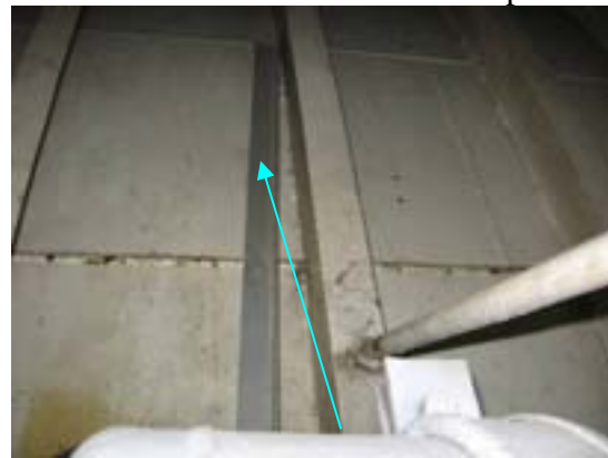
Plate inserted from previous bottom damage
