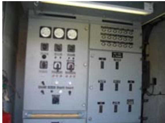
Emergency switch gear
