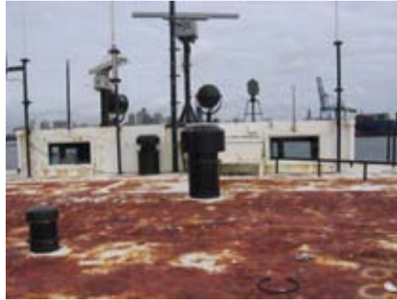
Antennas and searchlights and Housetop corrosion
