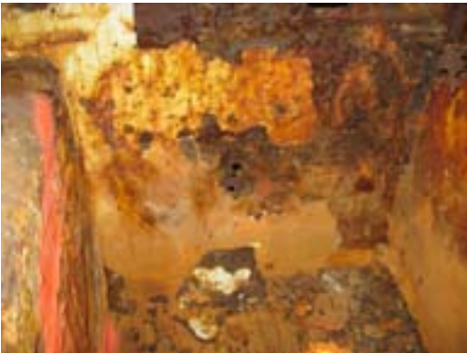
Holes in floors
