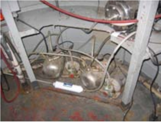
Galley service equipment
