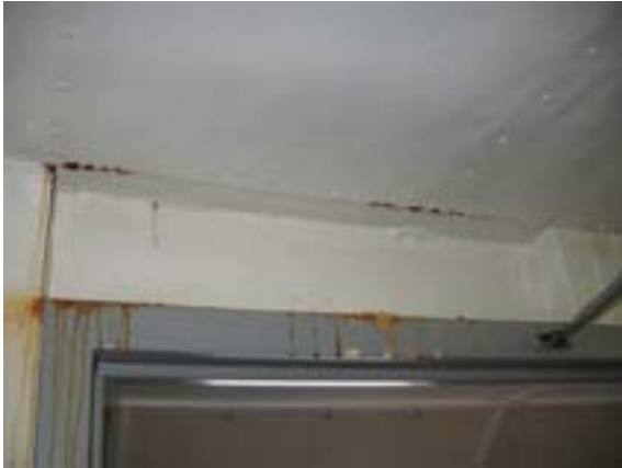
Leak from boat deck
