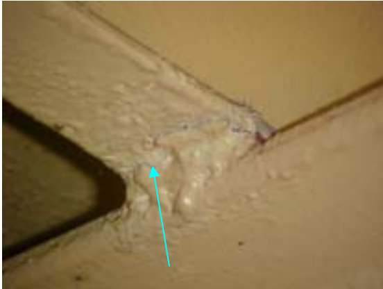
Crack in deck beam weld
