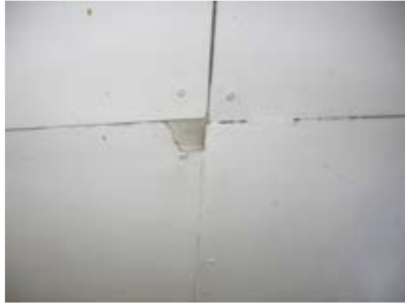
Asbestos ceiling in salon
