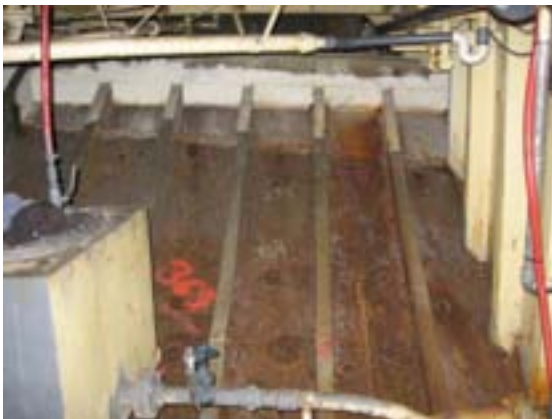
Coating Failure – active corrosion
