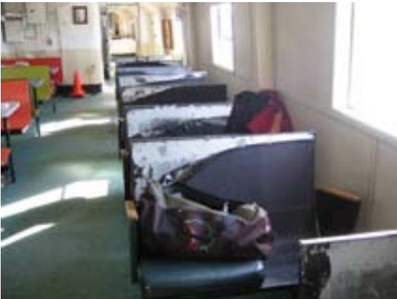
Worn out interior seating
