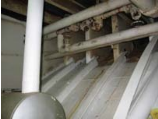
Coating failure in overhead
