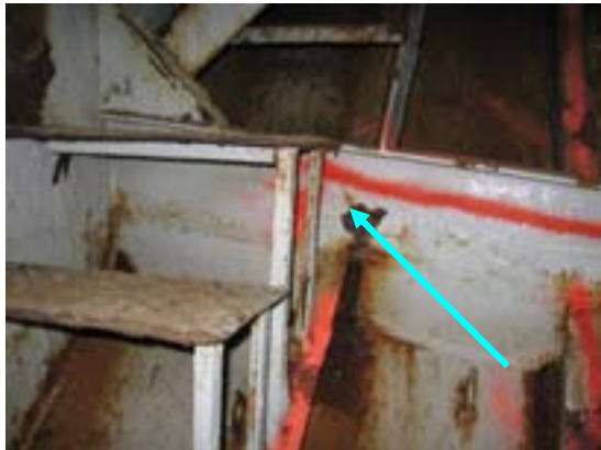
Hole in girder
