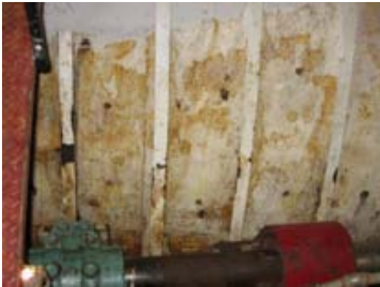
Coating failure – poor surface preparation
