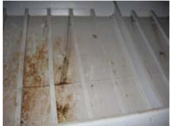
Localized coating failure
