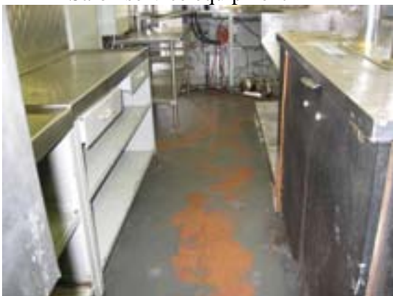
Worn deck in food service area
