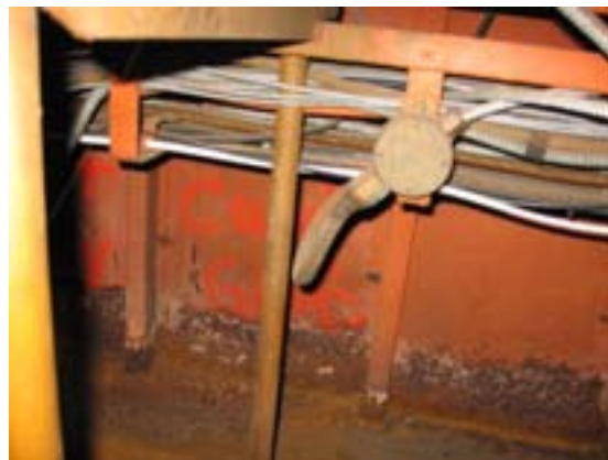
Corroded steel and coating failure
