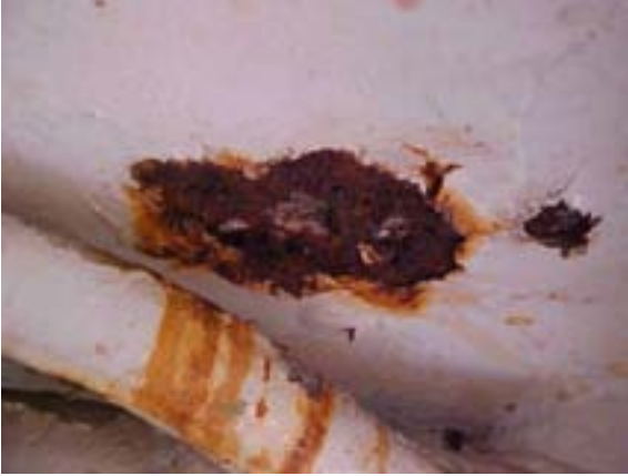
Hole in boat deck under salon
