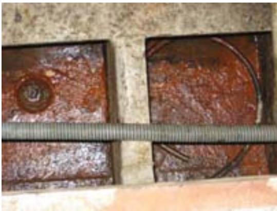
Corroded bottom plates
