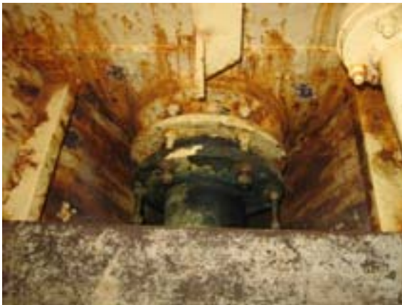
Wasted Steel bulkhead #47 aft
