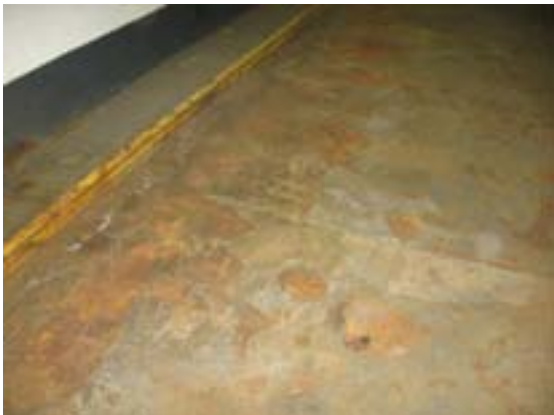
Significant coating failure
