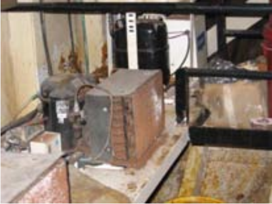
Corroded refrigeration compressors
