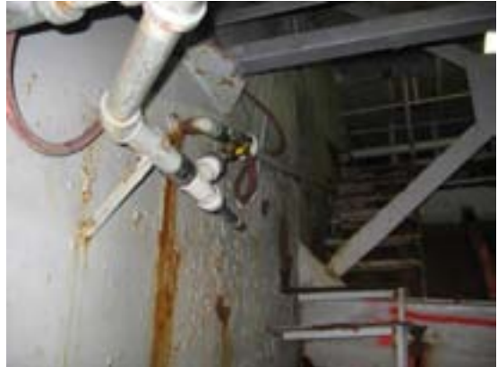
Wasted and buckled bulkhead #24 aft
