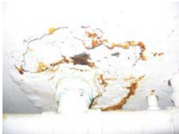
Deck wasted through at toilets
