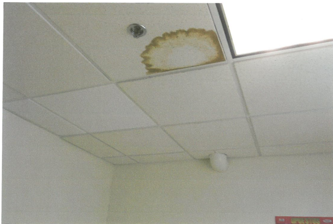
8: Stained ceiling tile (Spanish)
