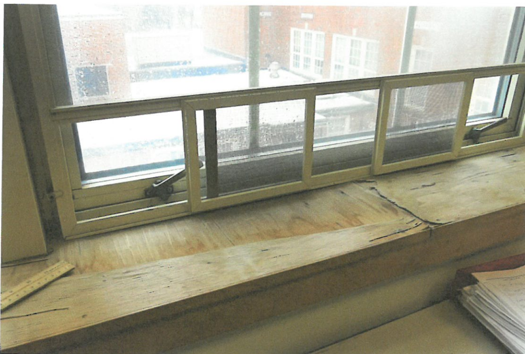
7: Delamination of window sill (rm 318)
