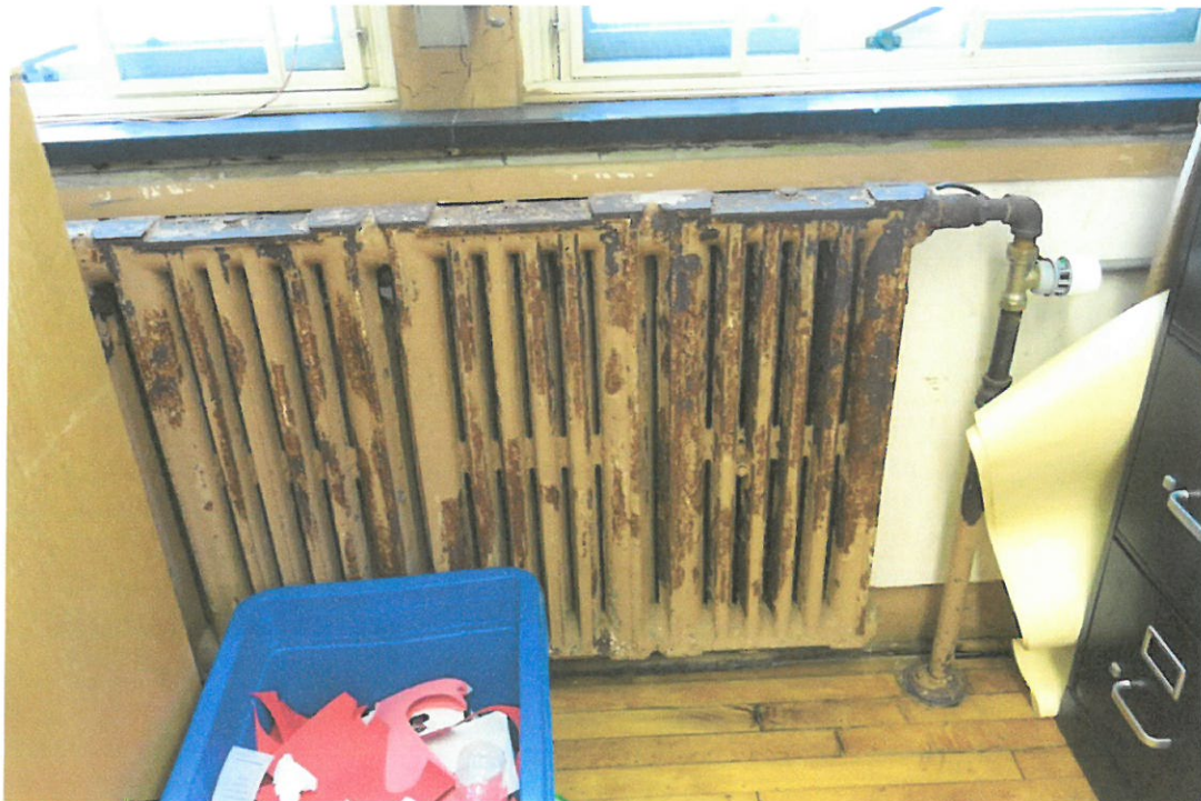
14: Rusted radiator with damage to wallboard behind the radiator (rm 201)
