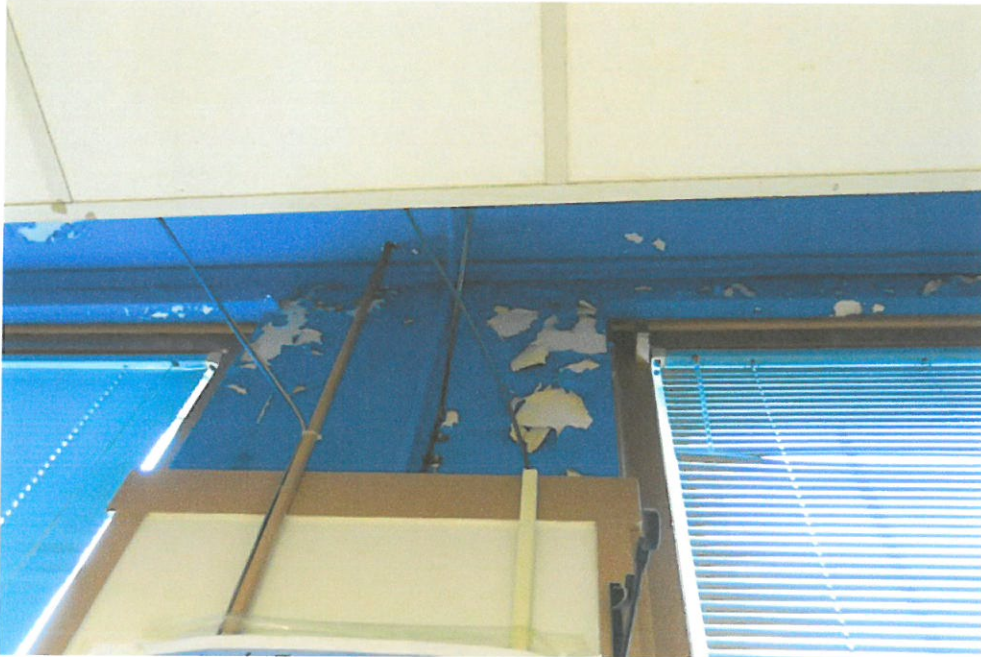
1: Evidence of water damage to paint near classroom windows (room 312)
