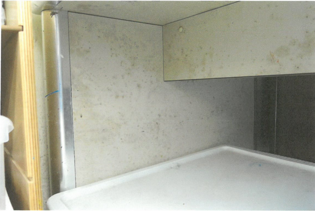
15: Mold/mildew growth (Art room)
