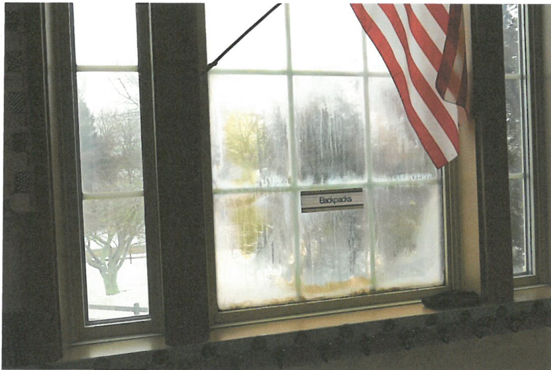
12: Condensation in window (rm 201)
