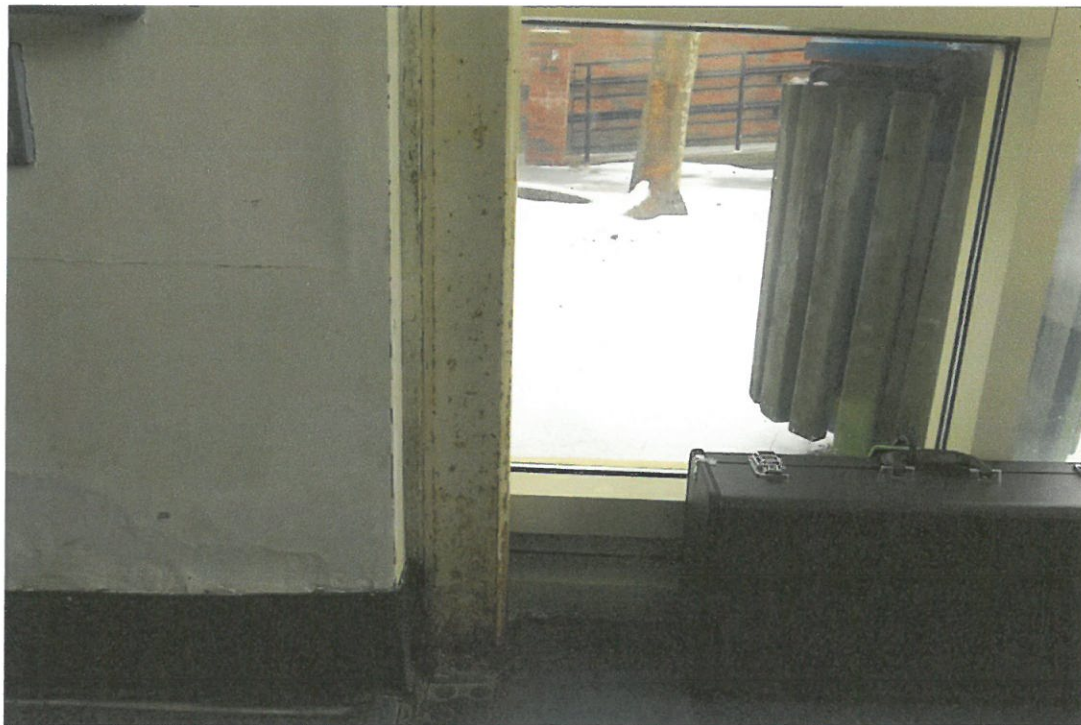
10: Rust on post near window (entrance with barrel arch)
