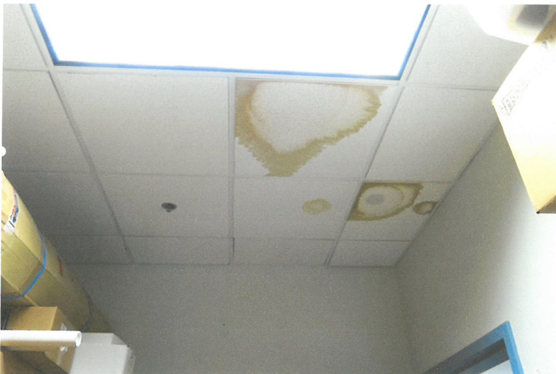
9: Stained ceiling tiles (rm 319)
