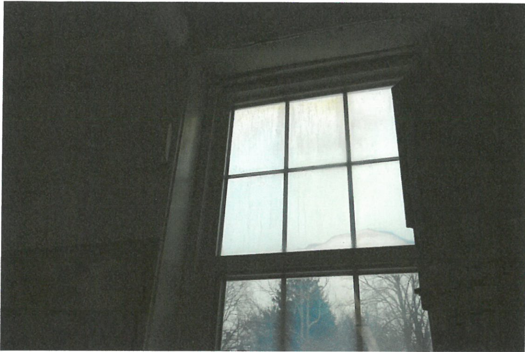
11: Condensation in window (Art room)
