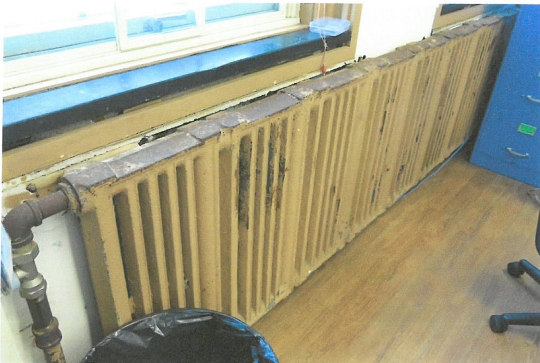
5: Damage to wall behind radiator (rm 216)
