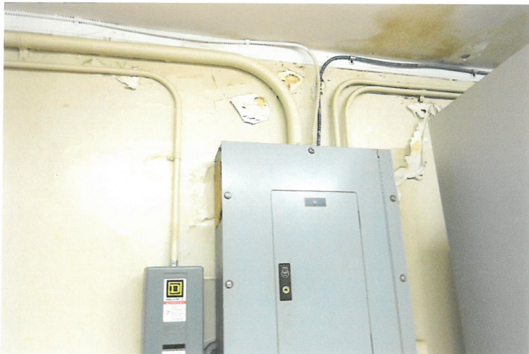
2: Water damage to kitchen wall near electrical box
