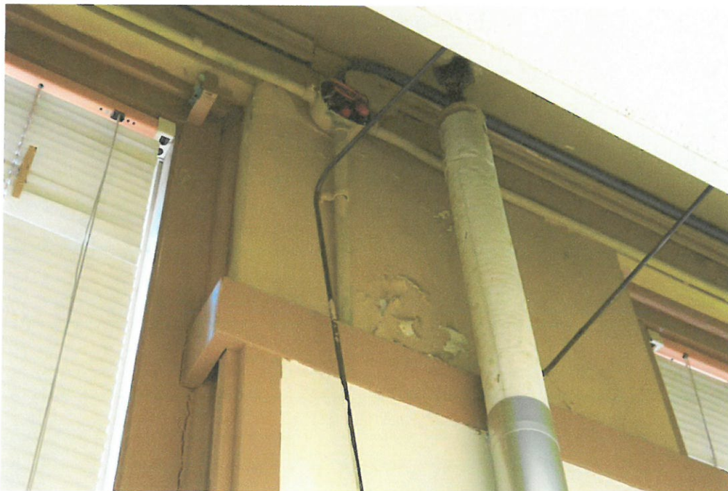
4: Evidence of water damage near open electrical box (Math Vocabulary)
