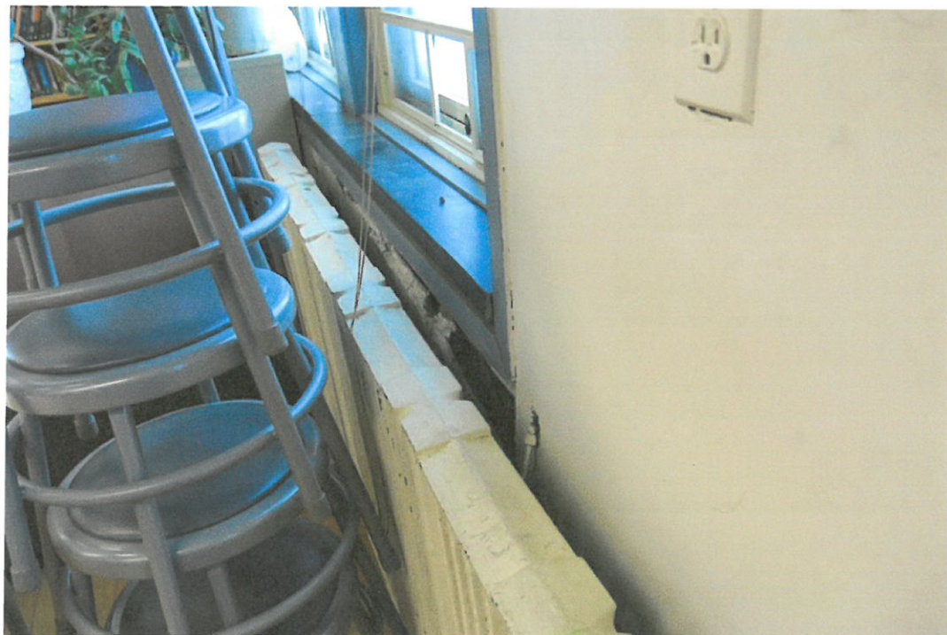
6: Damage to wall behind radiator (rm 313)
