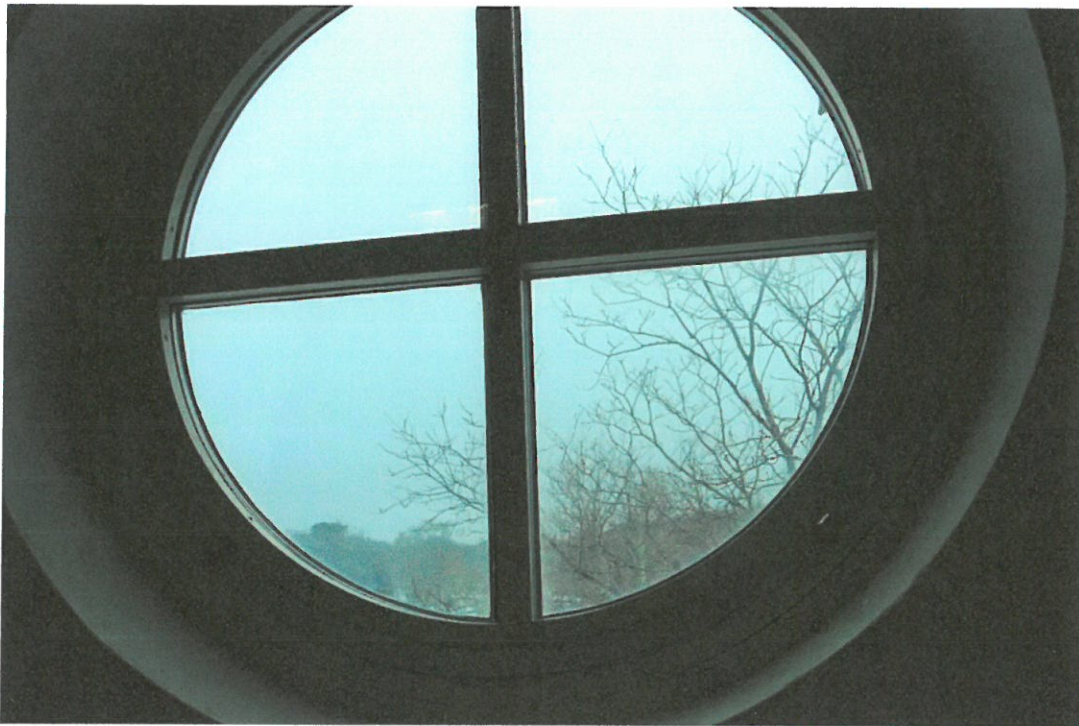
13: Break in window seal at 4:00 position (teachers' room)
