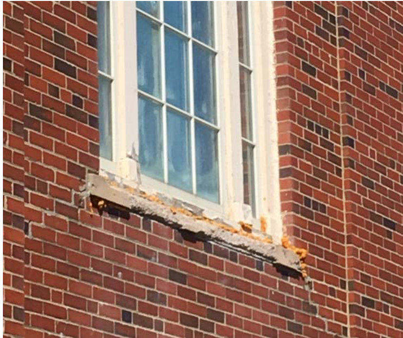
Damaged window frame and sill with spray foam insulation
