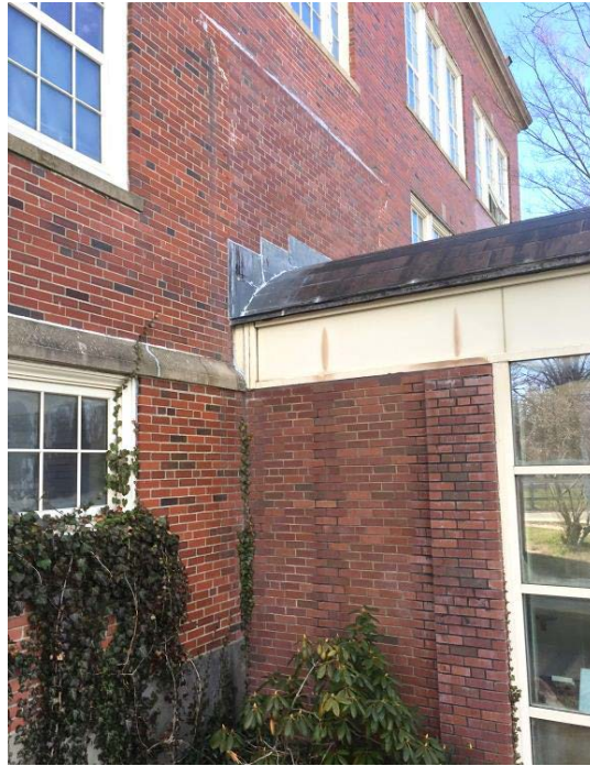
Sealed opening in brick above the east entrance (Note sealant and blackened brick above entrance roof)
