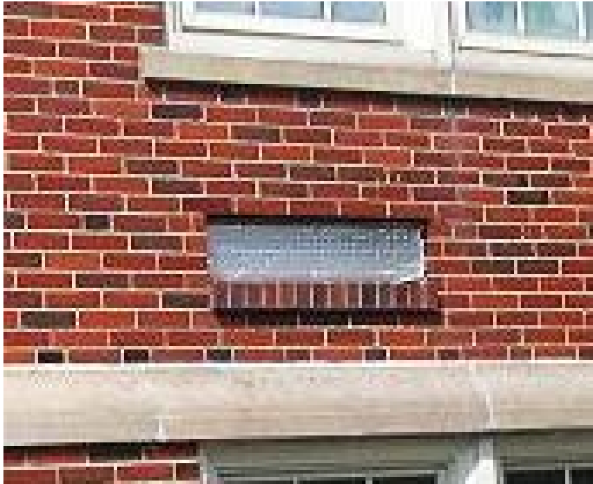
Sealed univent fresh air intake
