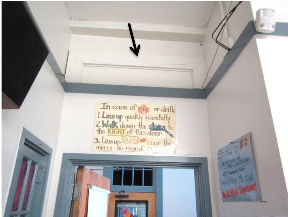
Sealed transom (arrow)
