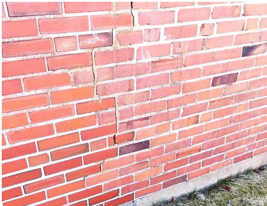
Gymnasium wing exterior wall cracks
