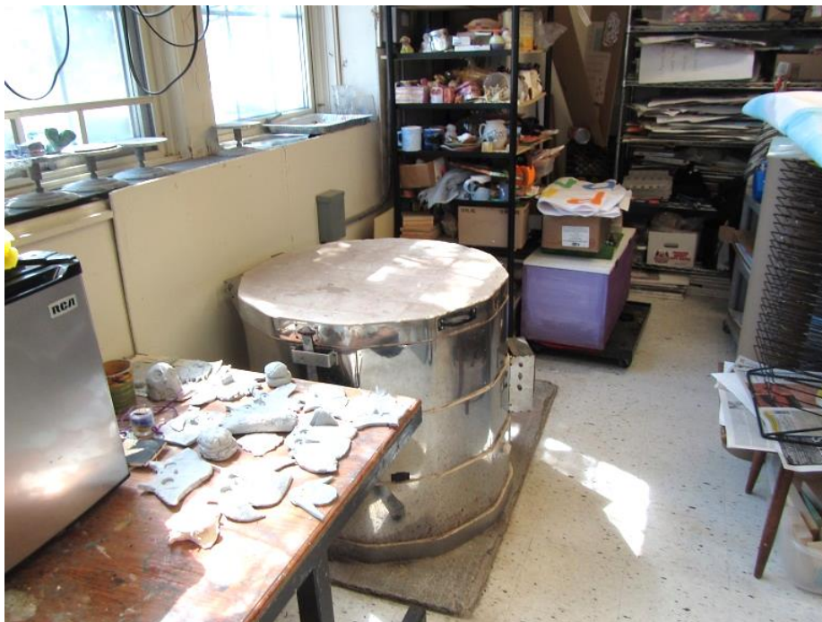
Kiln in art room with no dedicated exhaust vent
