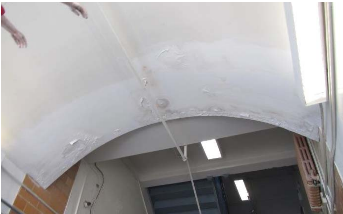
Water damage inside the east entrance
