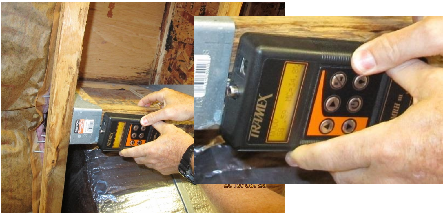
Elevated MM reading of 34+% MC indicating a still active leak associated with exhaust penetration
