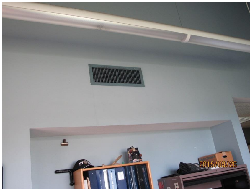
Clean grate in rear Officers Room
