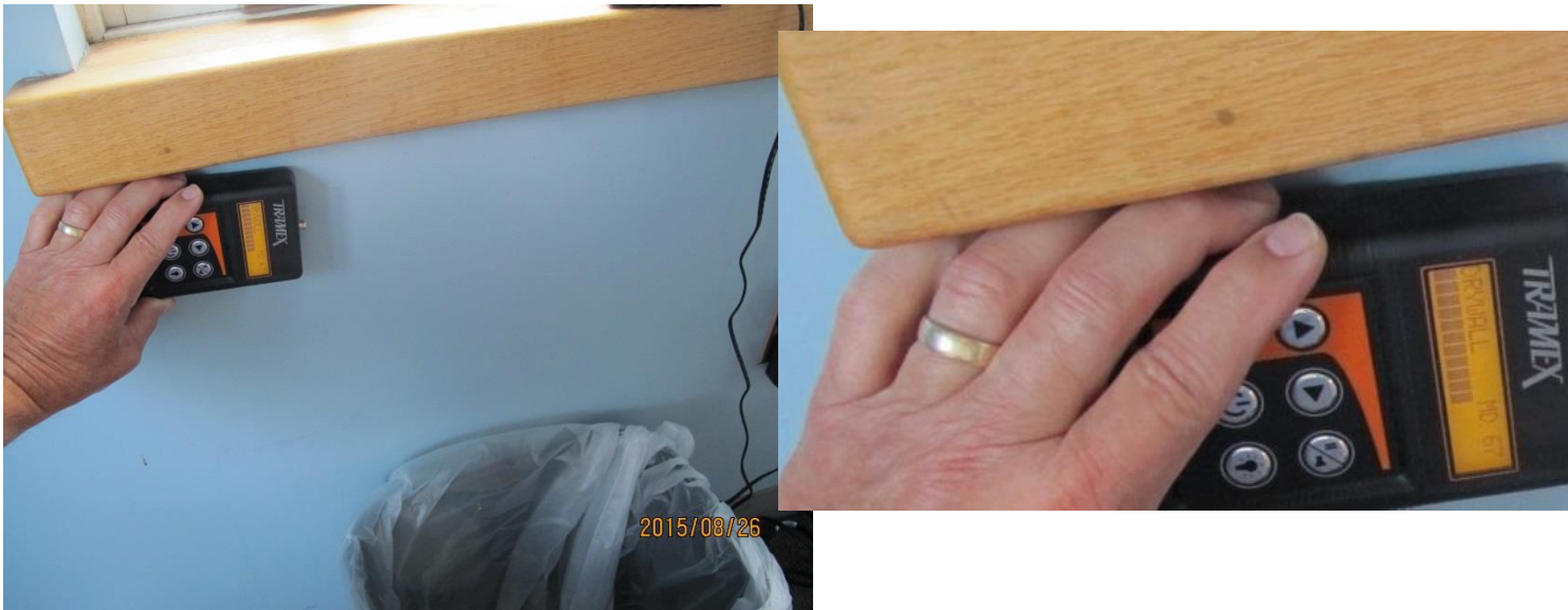
MM reading of 67% FS-DW under lower left corner of rear window in right side wall of rear Officers Room
