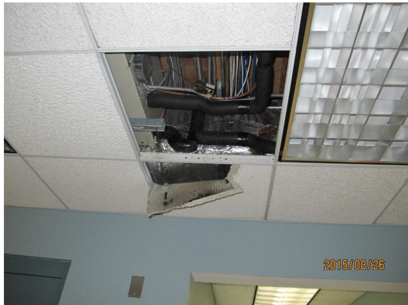
Ceiling leak in Briefing Room
