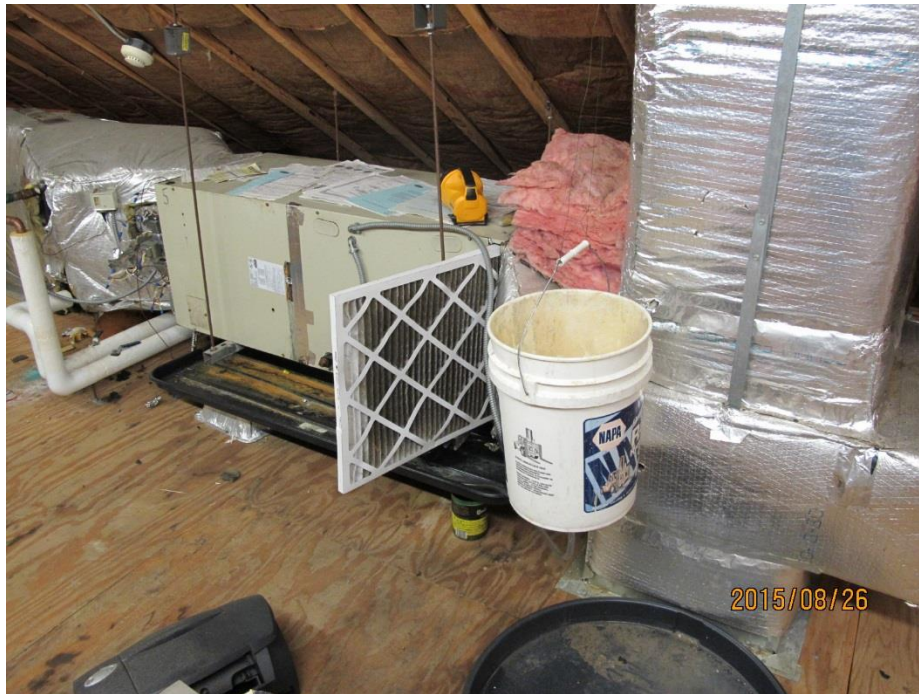
Dirty air filter for middle air handler in attic next to jury-rigged leak trap
