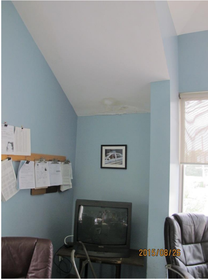
Water-damaged right, front wall (as viewed from the parking lot) in front Officers Room
