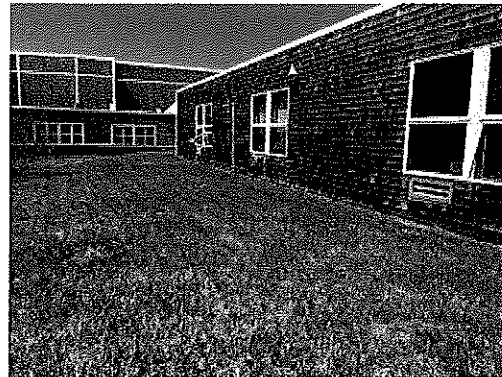
Covered Unit Ventilator Outdoor Intake Louvers
