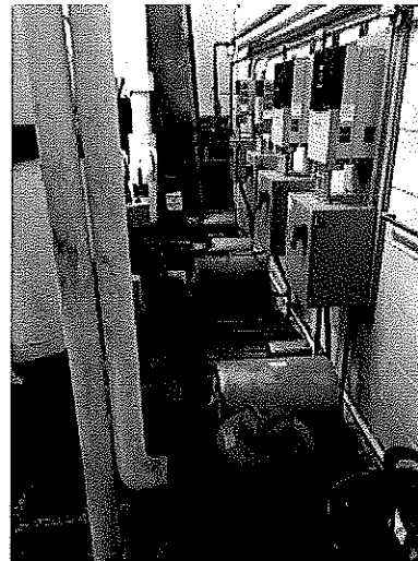
1994 Addition Hot Water Pumps
