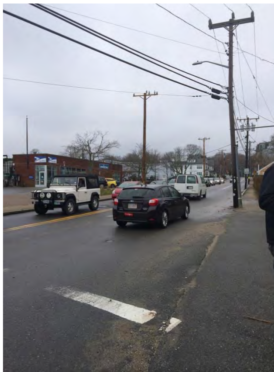
Faded pavement markings along the westbound lanes on Beach Street.
