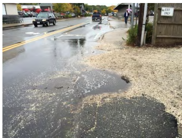
Poor stormwater management along Water Street.
